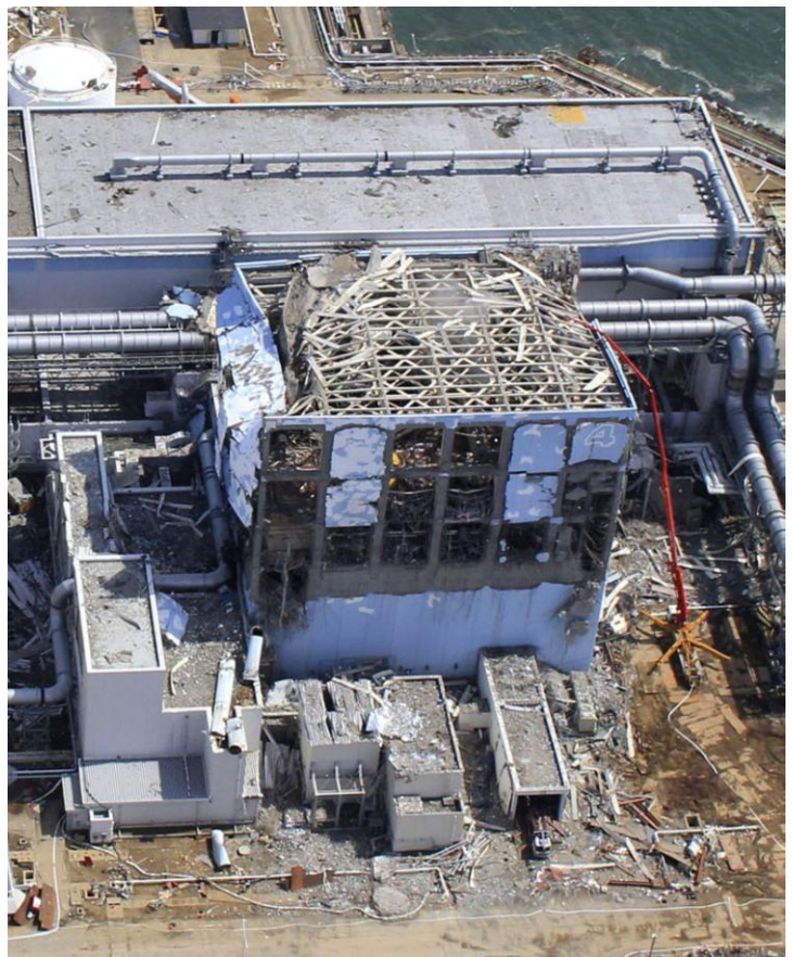
Figure 7: Fukushima Daiichi nuclear power plant's unit 4 reactor damaged by explosions and fires caused by earthquake and tsunami (Source: Air Photo Service)
